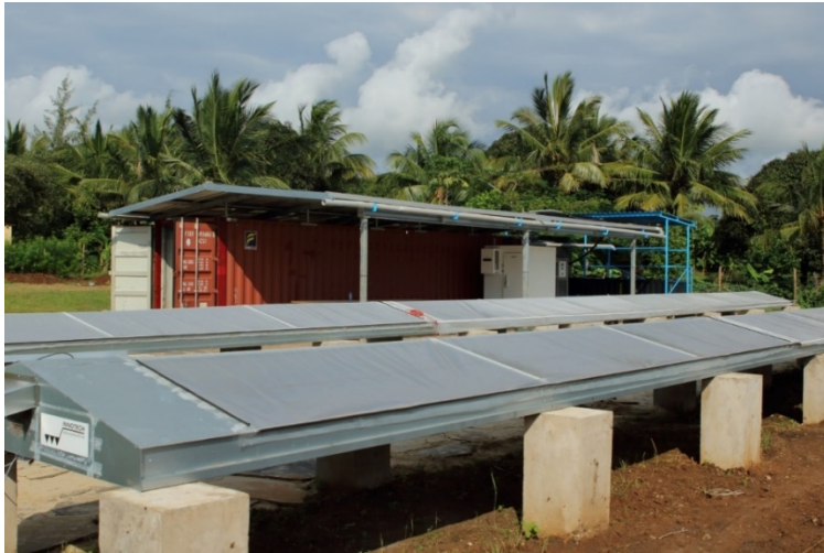
The SolCoolDry system consists of two tunnel dryers and a photovoltaic system (on the container roof) as well as the ice machine. © Fraunhofer ISE
