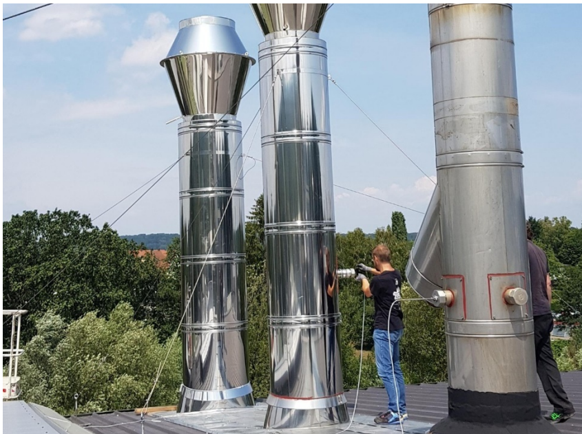
On-site at the demonstrator system of the industry partner Comet Schleifscheiben GmbH. The waste heat potential was determined for each chimney and the waste heat recovery was implemented at the one with most potential. ©Fraunhofer ISE
