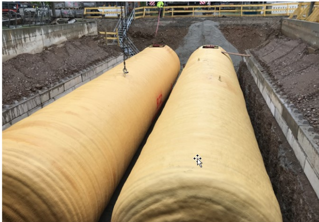
In the project, a cooling network and a cold water storage tank were installed at Fraunhofer ISE. ©Fraunhofer ISE
