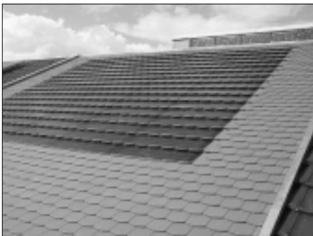
Fig. 2: Integration of PV roofing tiles into the roof of the "Butzweilerhof" Training Centre.
