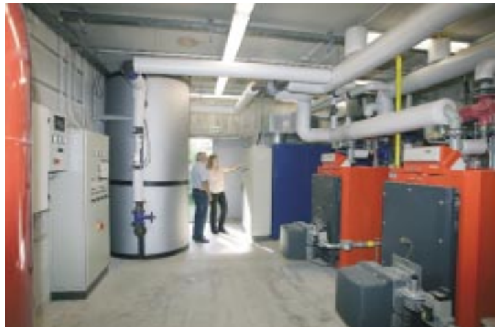
Fig. 1: The utility, MVV Energie AG, installed a CHP plant (at the back right of the photo) with peak-load boilers and a thermal buffer storage tank to supply heat and electricity to the ecological solar estate, "Am Steinweg" in Stutensee, near Karlsruhe. The system was extended with a photovoltaic system and a battery bank. Fraunhofer ISE optimised the system management with the PoMS energy management system. Photo copyright: MVV Energie AG
