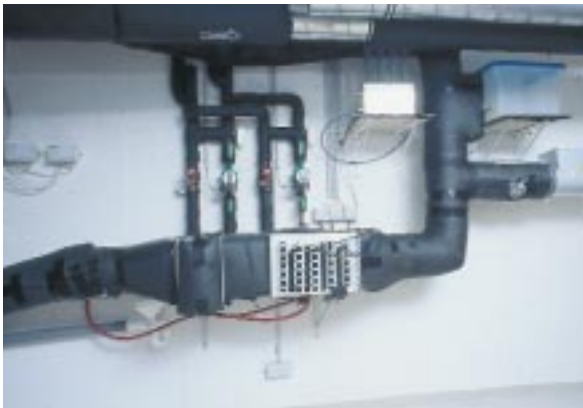
Fig. 2: Conditioning unit for outdoor air (insulation partly removed): The outdoor air flows in from the lower left through the pre-cooler/dehumidifier and the low-temperature chiller, then upwards to the ultrasonic humidifier and air heater. Two air currents can be separately conditioned as supply air and as a second heat source.
