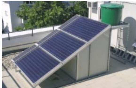
Fig. 3: First test model of the compact seawater desalination system that is powered exclusively by solar energy, which was set up on the roof of Fraunhofer ISE in October 2004. Thermal energy for the membrane distillation is provided by three solar collectors. The pump and the control components are powered by a photovoltaic module.
