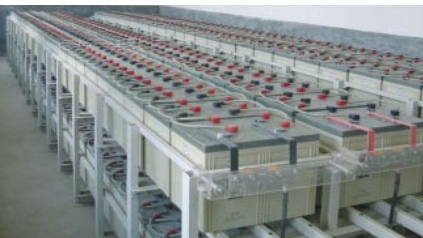
Fig. 2: In almost all Chinese village electrification systems, as here in Dousong village, only lead-fleece batteries are operated, with a system DC voltage of 220 V. As individual cells of this battery type are prone to break down unexpectedly, the systems are monitored continuously.
