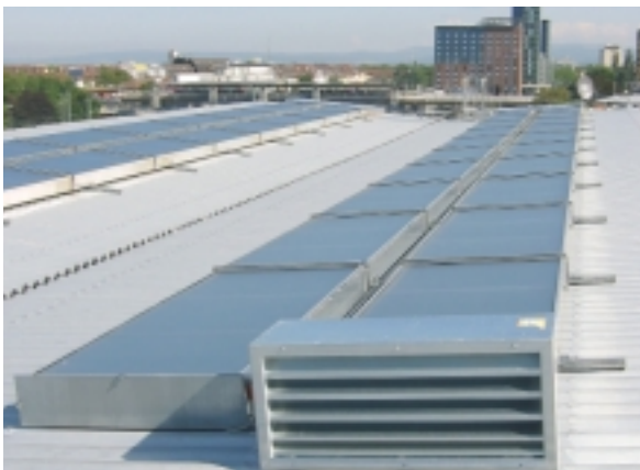
Fig. 2: Shutter box (in the foreground) to disconnect a collector string of the solar air collector system on the roof of the Regional Chamber of Commerce (IHK Südlicher Oberrhein) in Freiburg. The thermal driving power can be regulated by disconnecting individual collector strings, allowing unnecessary heat transfer to the room air to be reduced when the inlet air flow rates are low under partial load conditions.
