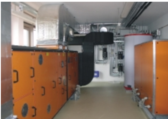
Fig. 1: Plant room with the Menerga system. To the right are the two tanks for the salt solution in the foreground and the solar buffer tank in the background. The ventilation equipment can be seen to the left. Solar energy is used in summer for air dehumidification and in winter for heating.
