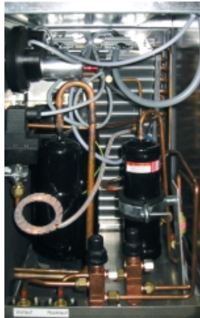
Fig. 1: Exhaust-air heat pump in an opened compact ventilation unit (required floor area: 0.5 m 2 ). It uses the sensible and latent heat of the exhaust air as a heat source and meets the entire demand for space heating and domestic hot water in a passive house. Conversion to refrigerants without greenhouse gases (FHC) is a goal of our development work.
