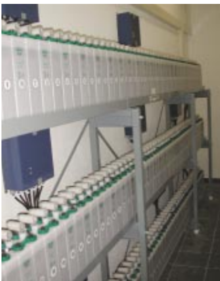
Fig. 3: Uninterruptible power supply (UPS) at the Ruit tram stop in Stuttgart.
