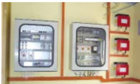
Fig. 2: View into the plant room with switchboxes and inverters. The switchboxes contain data loggers, all power meters and some of the inverters.
