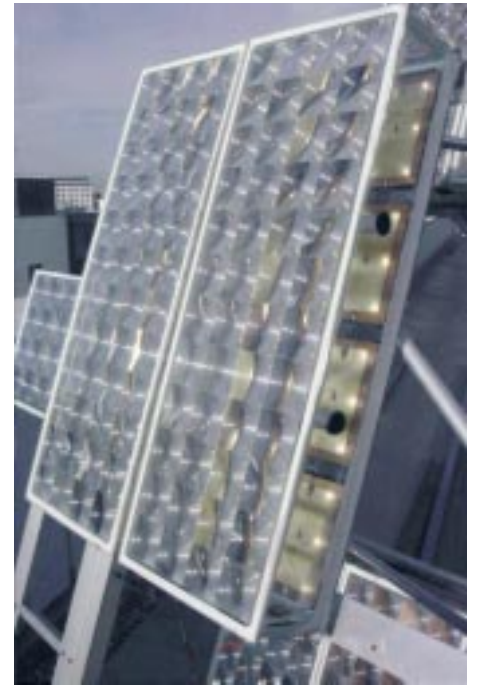
Fig. 4: FLATCON® modules mounted on the tracker on the Fraunhofer ISE roof.
