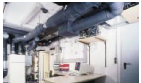
Fig. 3: Automated test stand for simultaneous measurement of two ventilation units with integrated exhaust-air heat pumps.
