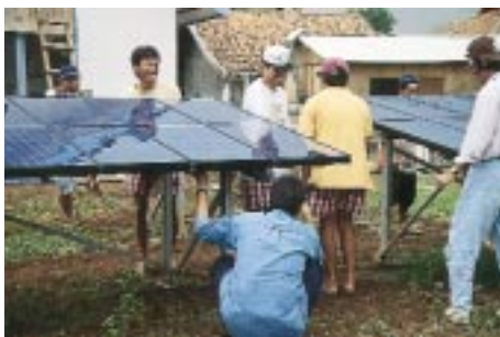
Fig. 1: Installation of a photovoltaic hybrid system in Indonesia.
