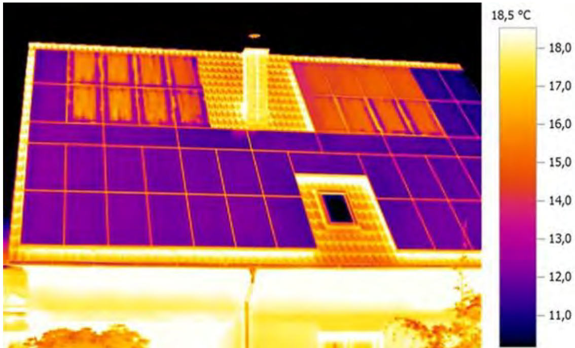
Figure 2-30: IRT image of a PID-s affected rooftop system with applied current during the night. In this case, the cooler cells are the PID-s affected cells [58].
