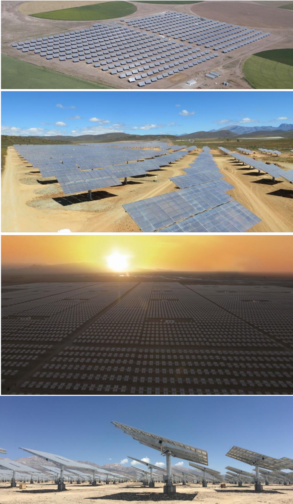
Figure 3: Examples of large CPV power plants. From top to bottom: 30 MW plant in Alamosa, Colorado, USA (© Amonix); 44 MW in Touwsrivier, South Africa (© Soitec); 140 MW in Golmud, China (© Suncore); a recent installation from 2016, 12 MW in Delingha City, China (© Redsolar).
